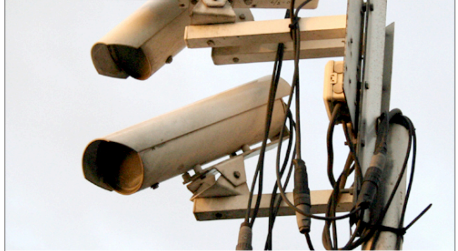
Video surveillance (CCTV)
